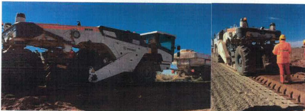
e. Compaction the milled mixture by using a compactor with vibratory sheepfoot or steel drum roller for achieving the required compaction
