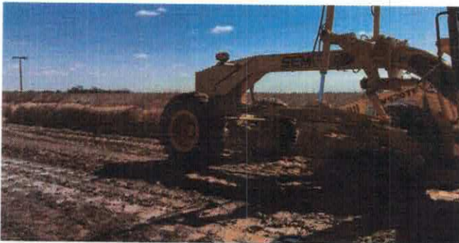
g. Final static and dynamic compaction of the fine level by using a steel drum roller
