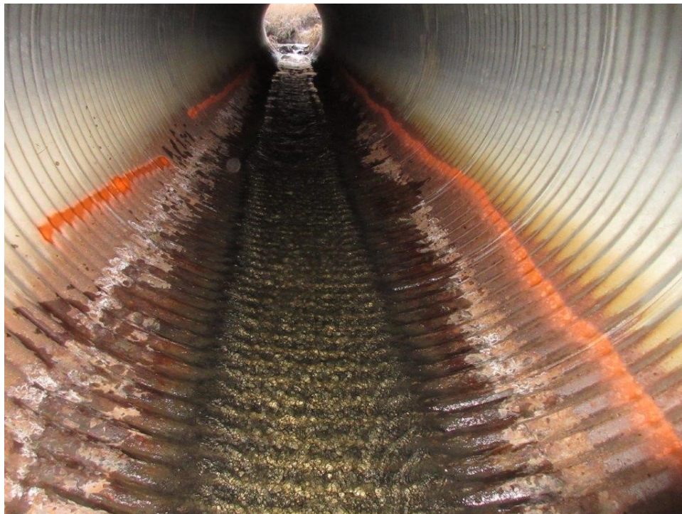
6. Looking U/S through barrel from Ring 2 near inlet. Floor has severe lineal perforations occurring along both hunches (highlighted with orange paint).
