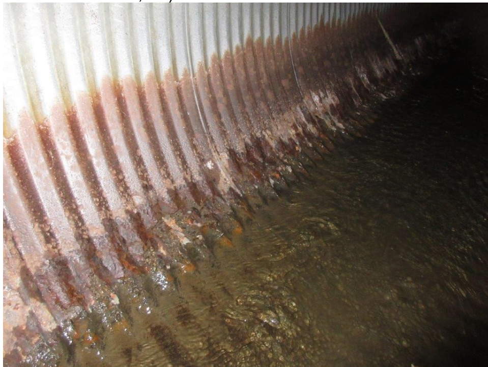
8. Typical continuous lineal perforations along west haunch.
