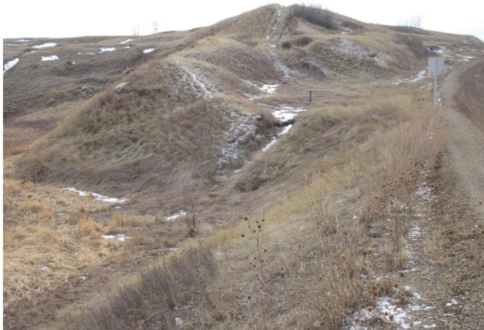
14. Minor erosion gully at the SW road embankment not currently affecting culvert.
