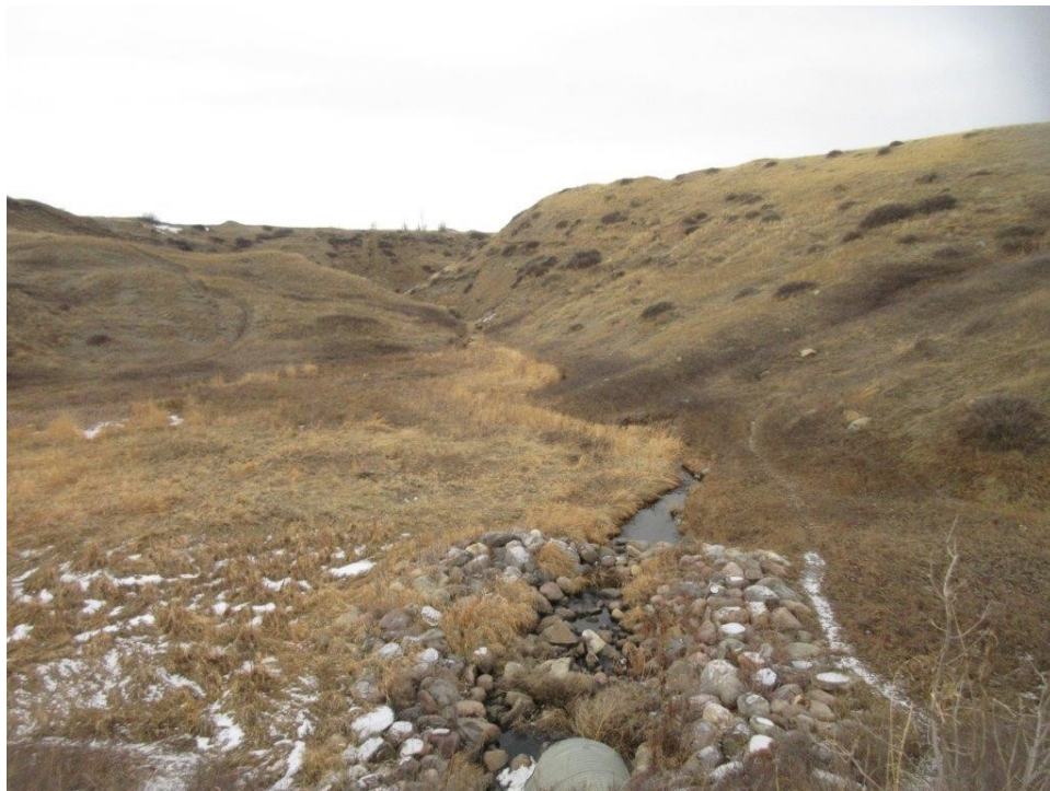
4. Channel alignment looking D/S. Outlet area is well protected by Class 2 rock rip rap.
