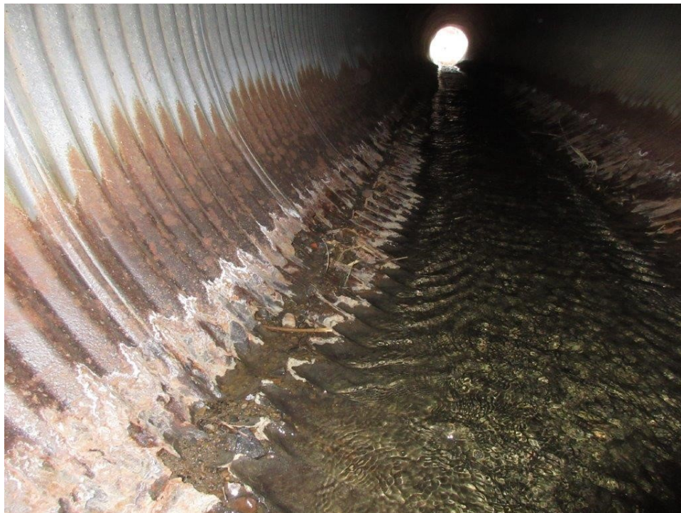
12. Visible backfill material and small voids at larger perforations in R4 and R5 along the west haunch.
