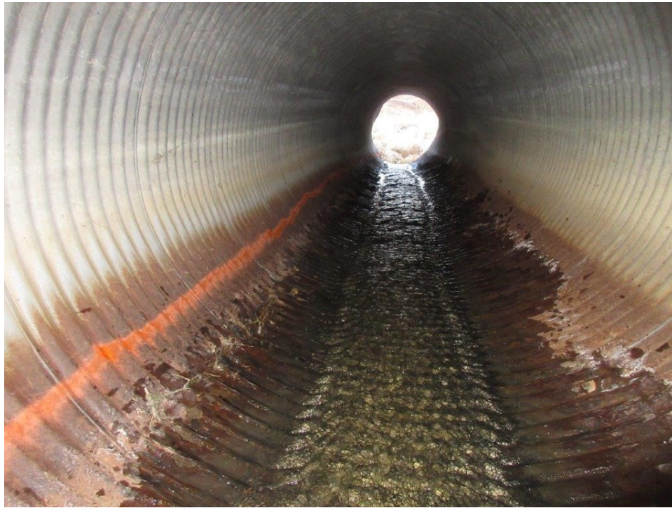
7. Lineal perforations are continuous for the entire length of the pipe (R1-R5) along the west haunch, and intermittent along the east side (R1 and isolated areas of R2-R4, R5).
