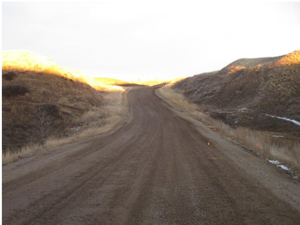
2. Road alignment looking east. Unknown utilities were in the process of being located and marked out during culvert inspection (flags on right shoulder).
