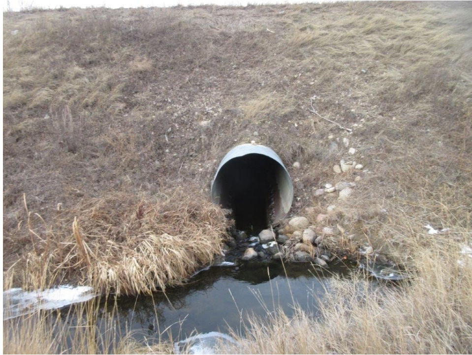
5. Looking north at inlet area. Minor erosion on both sides of the bevel currently appears vegetated and stable. Minimal rock protection.
