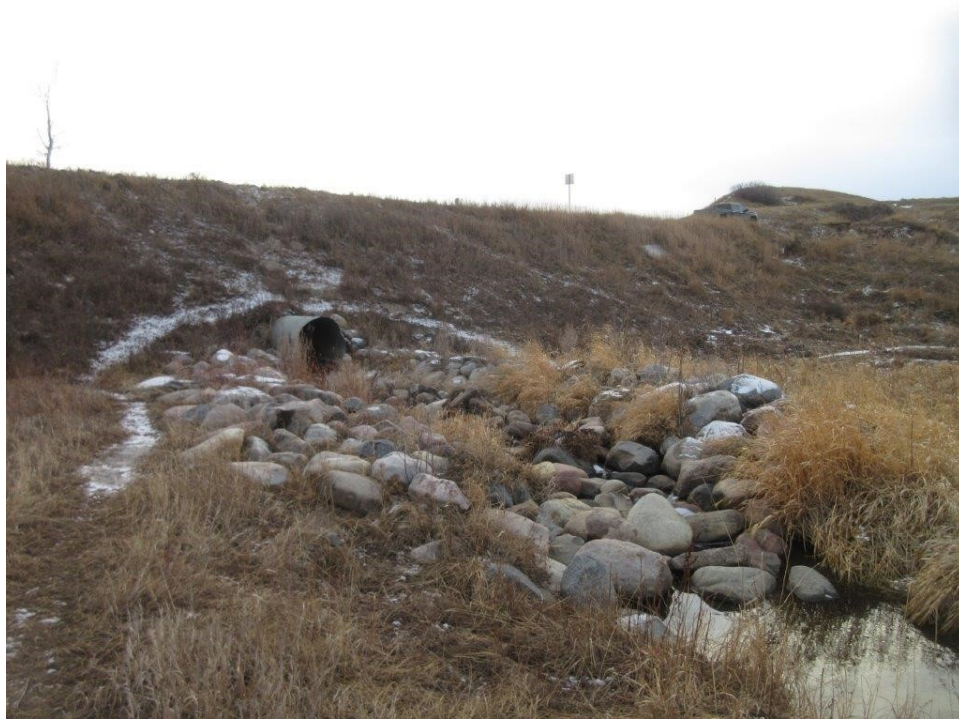
13. Outlet area undermining is due to piping and loss of backfill material related to perforations in barrel. Scour protection at outlet is in good condition and suitable for reuse.
