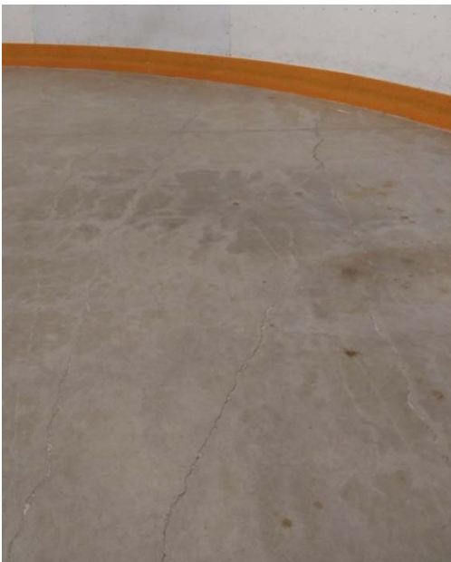
Photo 6: Slab crack near northwest corner.
