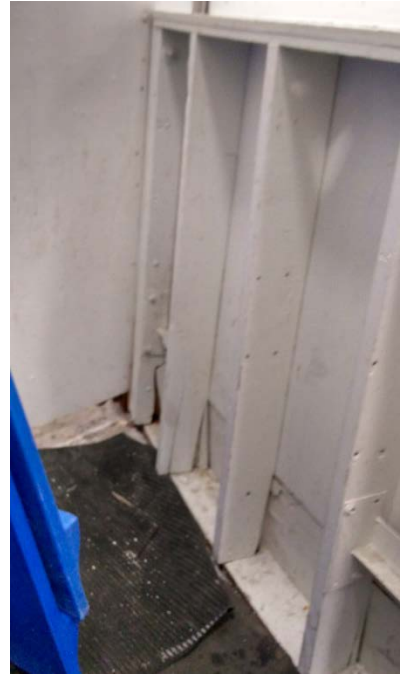
Photo 5: Damaged structural supports for the dasher boards.
