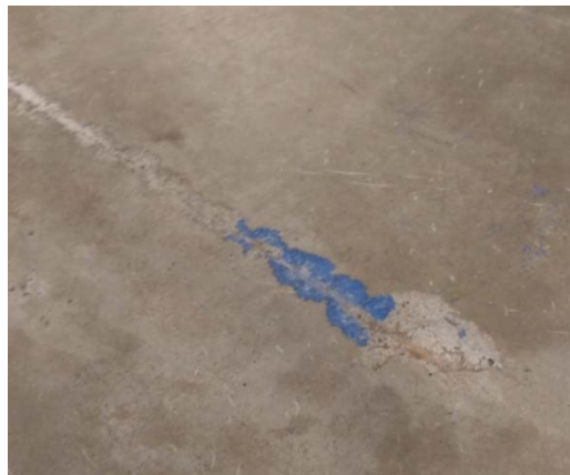
Photo 7: Exposed rebar in slab.
