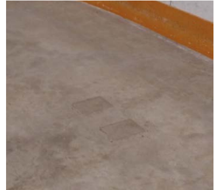
Photo 1: Showing location of curling hacks in slab from when space was used as a curling arena.
