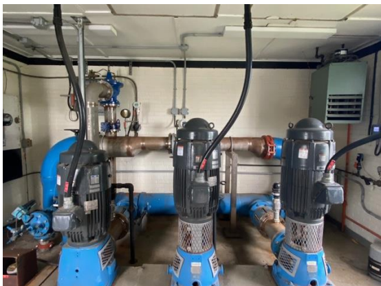
North Pump Station Upgrade
