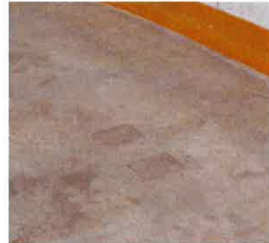
Photo 1: Showing location of curling hacks in slab from when space was used as a curling arena.
