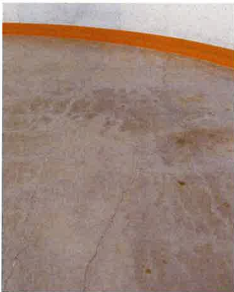
Photo 6: Slab crack near northwest corner.
