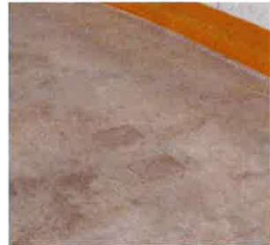
Photo 1: Showing location of curling hacks in slab from when space was used as a curling arena.
