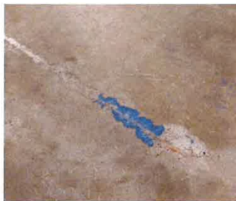
Photo 7: Exposed rebar in slab.
