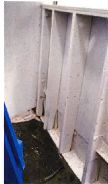
Photo 5: Damaged structural supports for the dasher boards.
