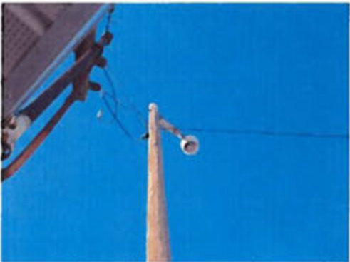
EXTERIOR ELECTRICAL SERVICE
