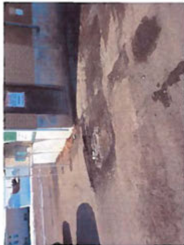
PAVEMENT CONDITION EAST BAY
