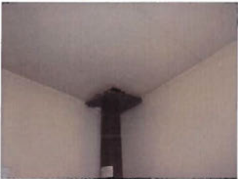
VENT STACK TO ROOF
