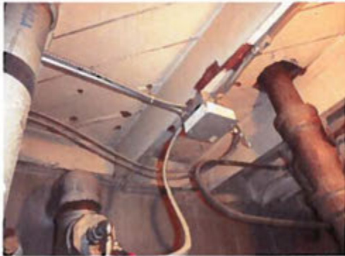
ELECTRICAL CONDUIT / JUNCTION BOX
