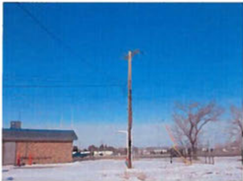
EXTERIOR ELECTRICAL SERVICE
