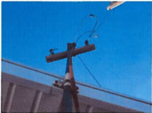
EXTERIOR ELECTRICAL SERVICE
