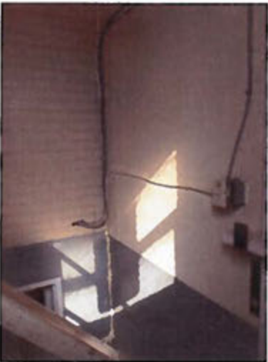
GENERAL ELECTRICAL - R EAR STAIRWELL
