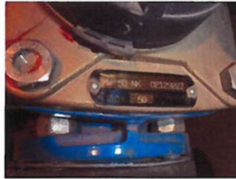
50MM FLOW METER
