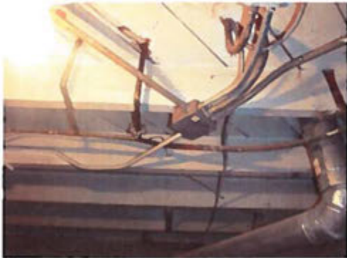
ELECTRICAL CONDUIT / JUNCTION BOX
