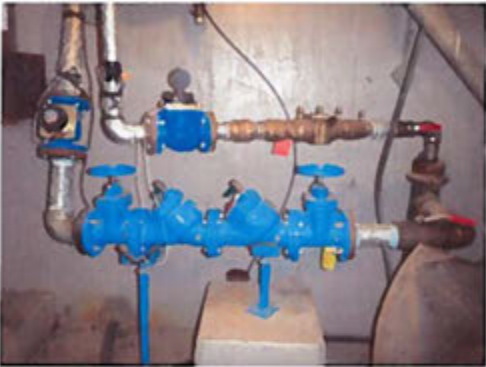
BACKFLOW VALVES AND FLOW METERS WEST WALL
