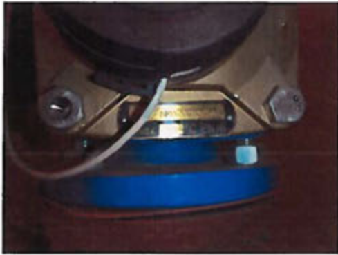
80MM FLOW METER
