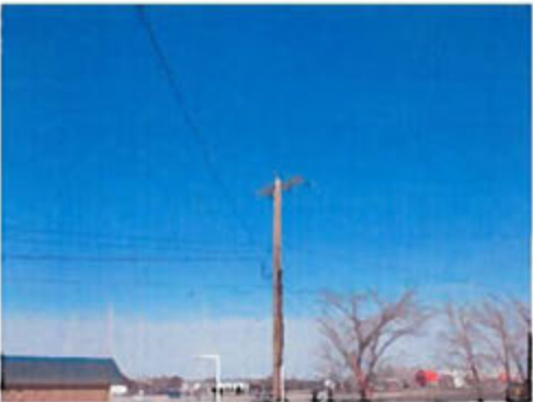
EXTERIOR ELECTRICAL SERVICE
