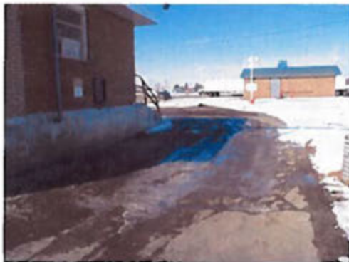
CONCRETE PAD CONDITION
