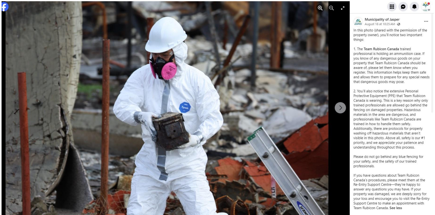
Safety was always the priority of all teams- Information Officers included. As residents re-entered, dangerous materials found in the ashes had to be communicated clearly. PC: Parks Canada
