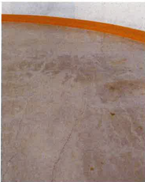
Photo 6: Slab crack near northwest corner.
