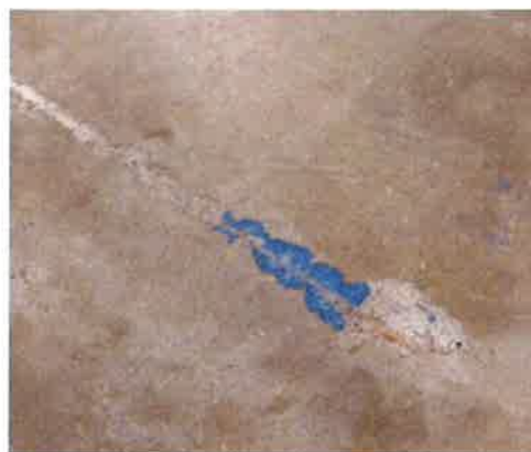
Photo 7: Exposed rebar in slab.
