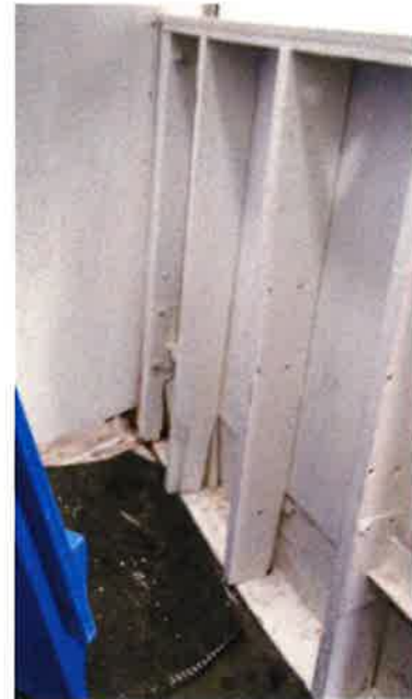
Photo 5: Damaged structural supports for the dasher boards.
