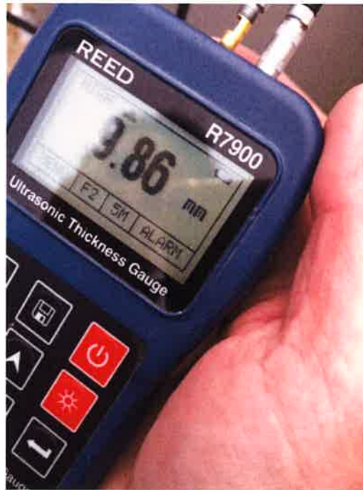
PHOTO 6 - HSS12X12 COLUMNS MEASURED TO BE 9.86MM (3/8" THK) USING REED INSTRUMENTS ULTRASONIC THICKNESS GAUGE
