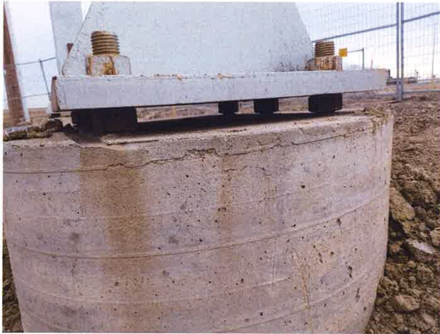
PHOTO 3 – U/S OF BASEPLATE IS SUPPORTED BY NUTS IN A STAND-OFF CONDITION.
