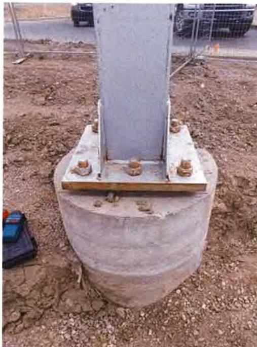
PHOTO 2 – CLOSER VIEW OF BASEPLATE AND EXPOSED PORTION OF PILE
